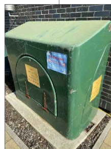
GAS EXTERNAL METER POSITION (WITHIN GRP ENCLOSURE) CW EXTERNAL ISOLATION POINT
